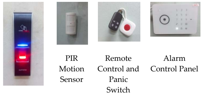
Figure 3.1a: Fingerprint Reader and alarm system
